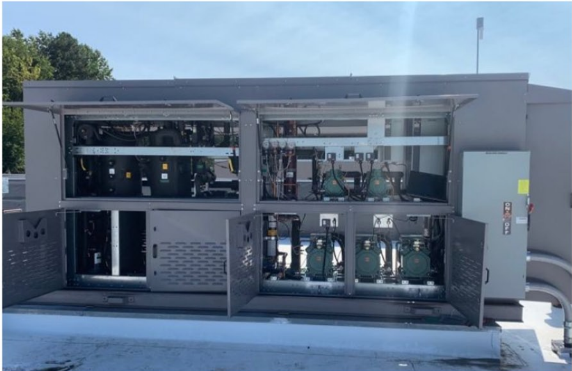
Transcritical CO 2 rack with FTE technology installed in the U.S.
